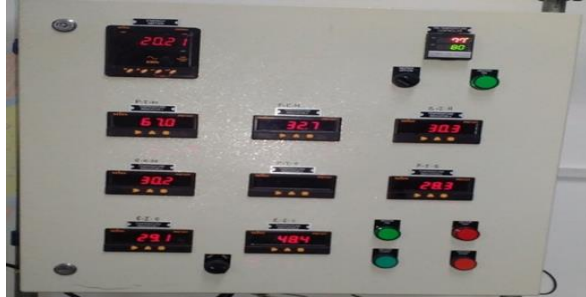
Figure 2 Control Panel and Display Board
