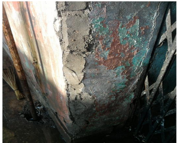
LEAKAGE OF WATER
