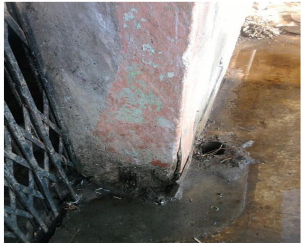
Horizontal And Vertical Cracks
