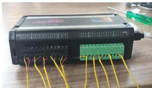
Fig 3.1.7: Data Acquisition unit and thermocouple connection to the channel
