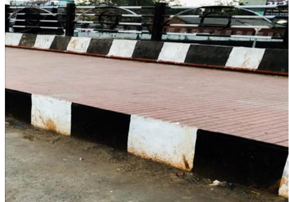
Figure 2 Inadequate height of footpath
