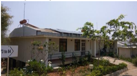
Fig 9: Solar panels on the roof
