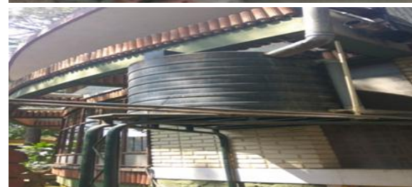
Fig 5: Rain water harvesting tank
