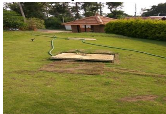
Fig 26: Rain water harvesting tank provided
