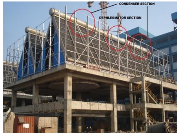
Figure 1.2 Air cooled condenser (UltraTech Cement Ltd.)
