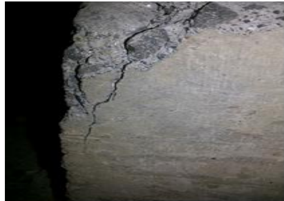
The cracks observed at the top of the column within ±2.5mm
