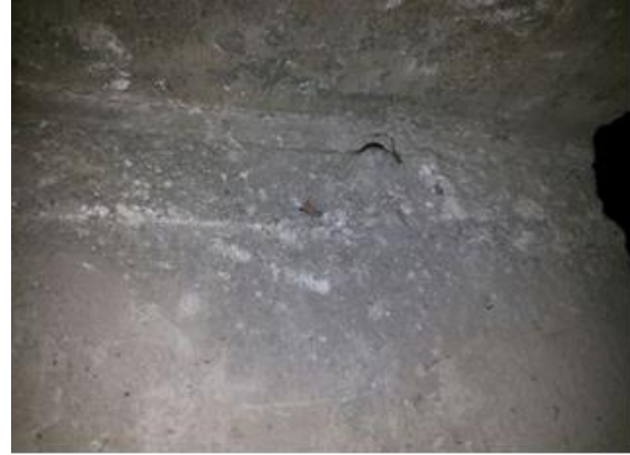
The cracks patterns observed at the time of testing within ±2mm in the junction of RC when applied a load on the top of the column and end of the beam (Jack 1 has 1000KN and Jack 500KN)
