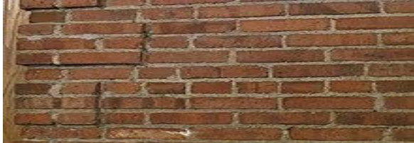
Fig No.1 – Brick masonry
