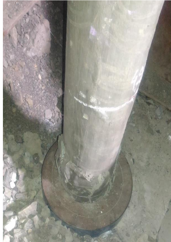
Fig.3. without wrap column failure
