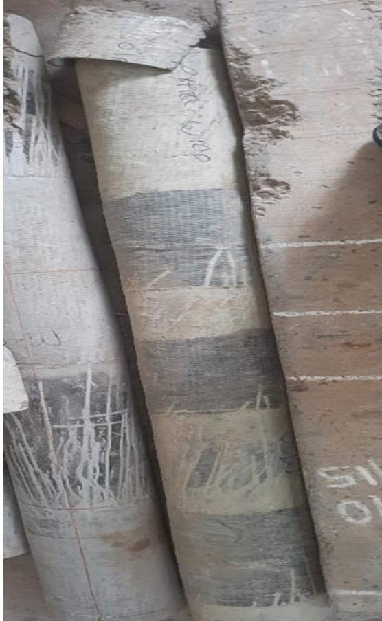
Fig.5. fully wrap column failure
