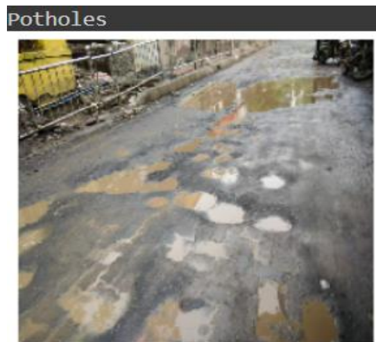
Fig. 4 Pothole Road detected (CNN).
