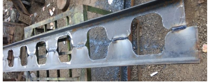
Figure No.2 Sinusoidal cutting of castellated beam II) Welding- Lastly welding of the web post back together at the high points is carried out with an automated submerged arc welding process.
