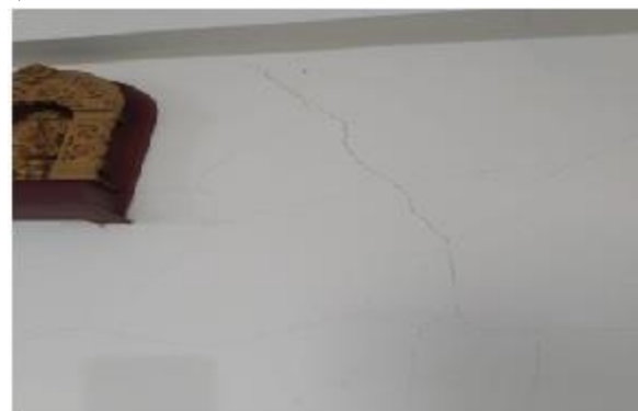
4) Internal Brick Wall Cracks, not for Structural Cracks
