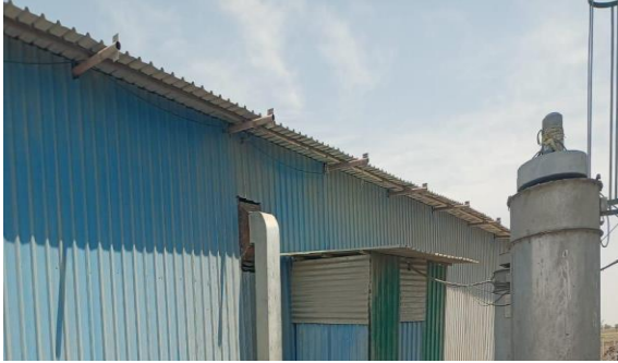
Photo 9, Dust duct installed inside cement go down to collect the cement dust directly into bags.
