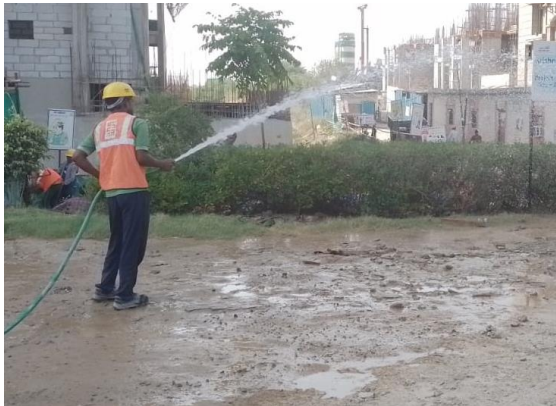
Photo4, The places not serviced by water tankers can be sprayed with water by hand.
