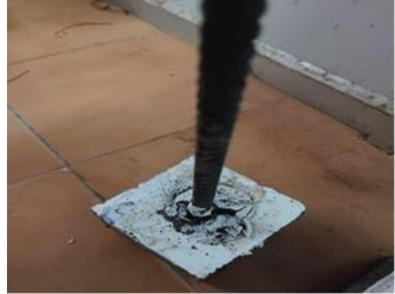
Figure (7) a) Pullout test setup b) Failure by steel bar pulling out of concrete
