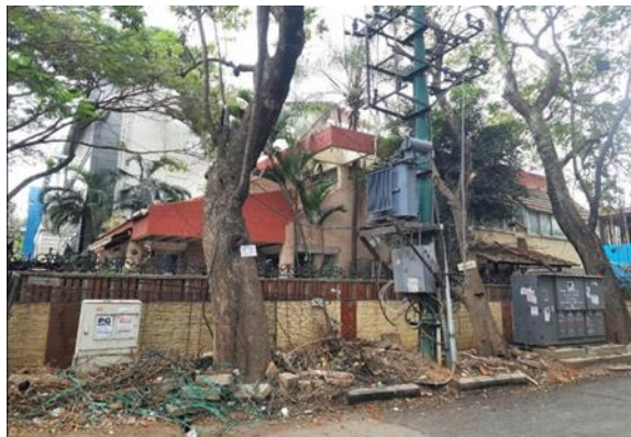
Figure 10. showing pole mounted transformer
