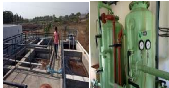
Sewage treatment plant Sand filter and carbon filter
