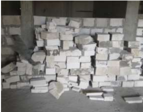
Fig. AAC Block wastage on site due to improper handling and placing
