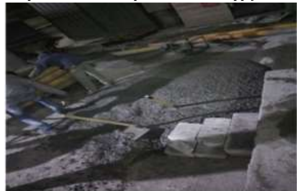
Fig. Concrete waste generated due to pumping line system
