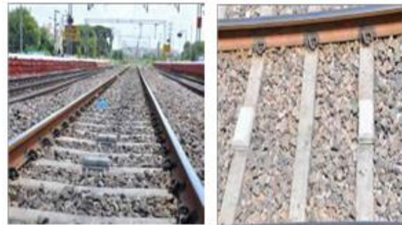
Fig 3: RFID Tags installation on tracks
