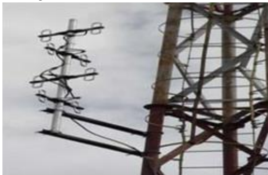
Fig: Station Radio Antenna
