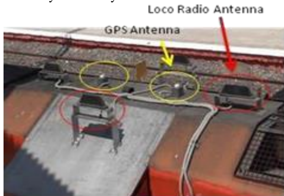
Fig: GPS Antenna & Loco Radio Antenna
