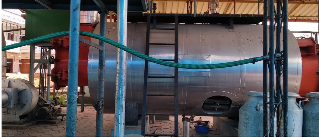
Fig(1)-Present Boiler plant in the company
