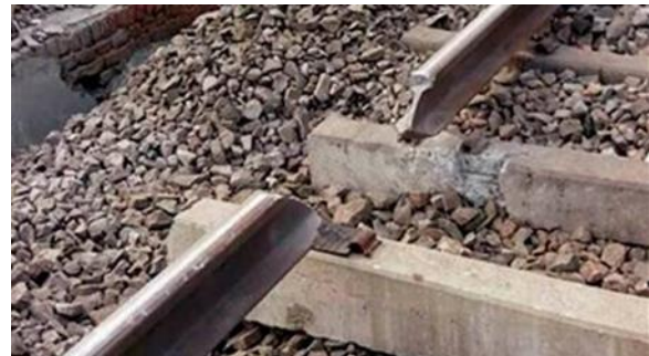
Fig. 1. Crack on Railway Track
