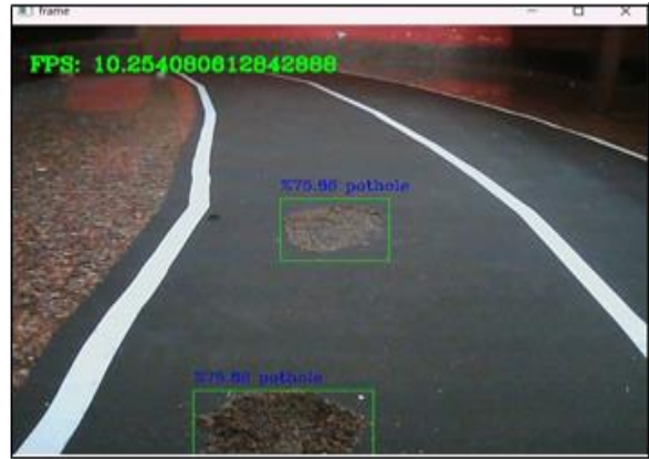
Fig .12.Detection of potholes
