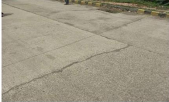
Figure No.3 Crack in direction perpendicular to traffic
