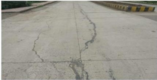
Figure No.4 Cracks on pavement repaired by filling them with bitumen
