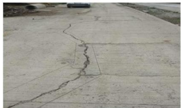
Figure No.2 Crack in the direction of traffic.
