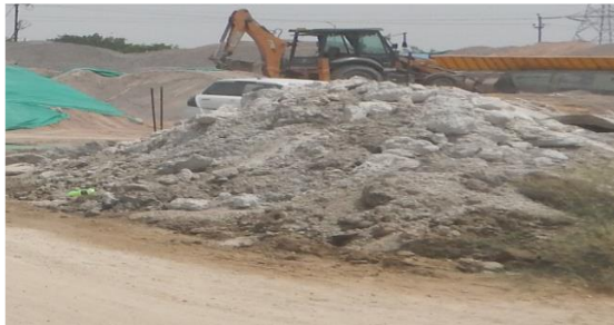
Fig 8 Improper Disposal of C&D Waste Leading to Dust Pollution
