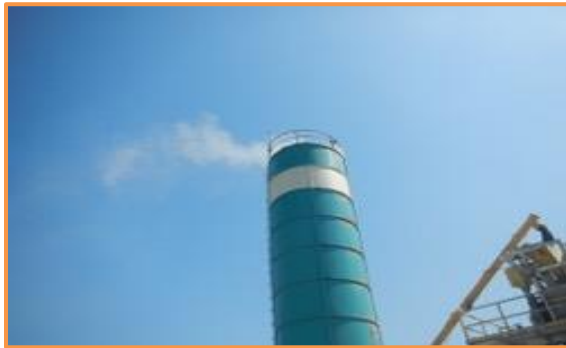
Fig 4 improper and irregular maintenance of cement silo vent air filter
