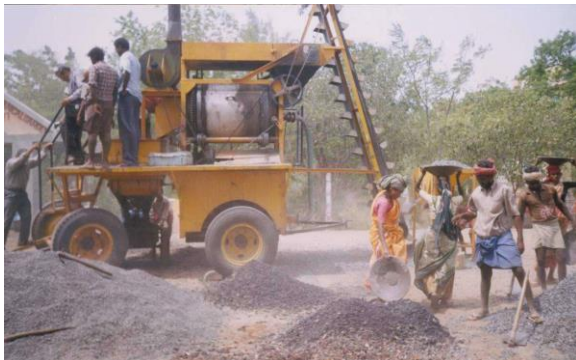
Fig. 4.4: Heating of Aggregate to 170° C in Mini Hot Mix Plant
