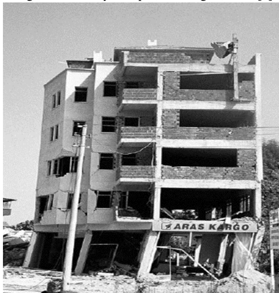
Fig.1.b Soft story failure, Bhuj 2001 [7].
