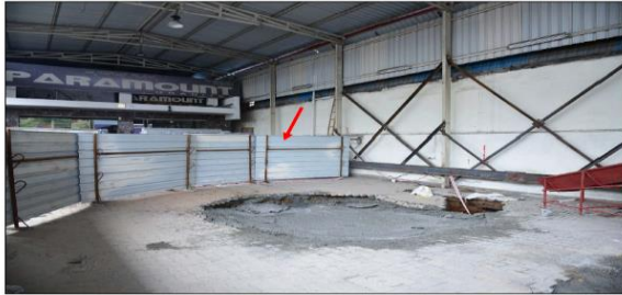
Fig. 16: Showing temporary arrangement near sink hole location
