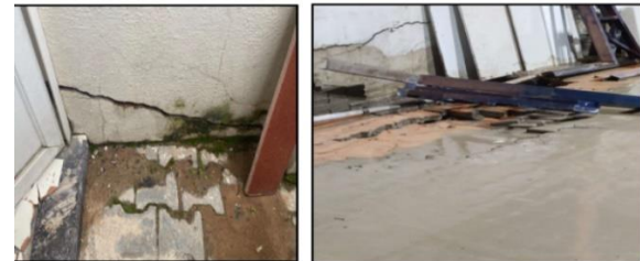
Fig. 14 Showing cracks on Paramount shop
