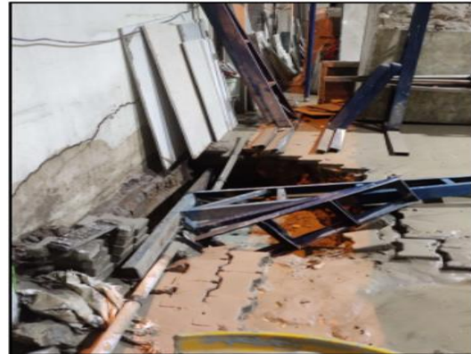
• Sink Hole occurred at "Paramount Marble Shop" on 20 July 2022 03:16 am at CH:8992.520m. (TBM S1259)
