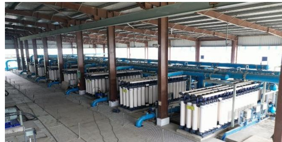
Fig 3 Ultra Filtration System
