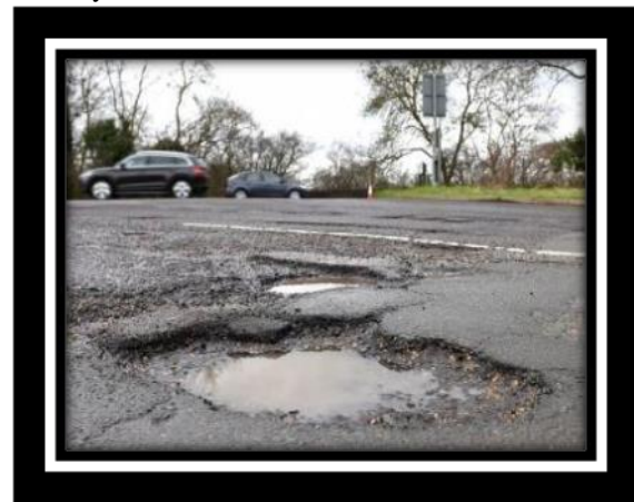
Figure 1 Conditions of roads with potholes.
