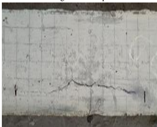
Fig 5 Crack in beam
