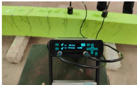
Figure.6 Crack depth Measurement by NDT
