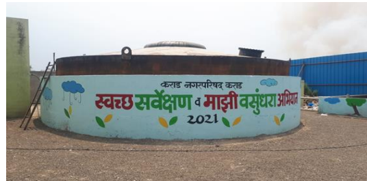
Fig.6 Digester into which Slurry is transferred
