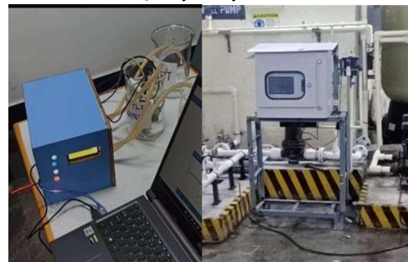
Figure.2 Real time water quality monitoring system
