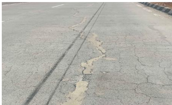
Fig. 2. Wear and tear of the polymer base epoxy sealant and cementitious grouting
