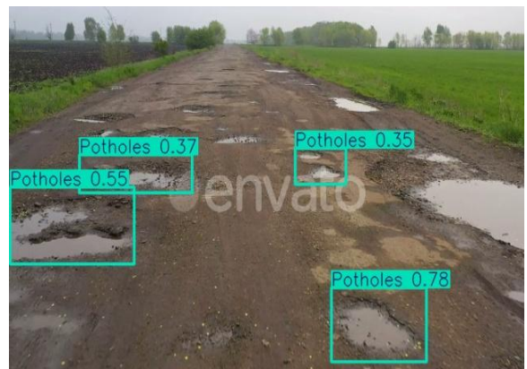
Figure 6: Outputs of Road Damage
