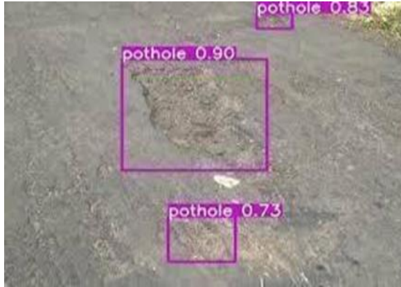
Fig 3. Pothole detection on Roads
