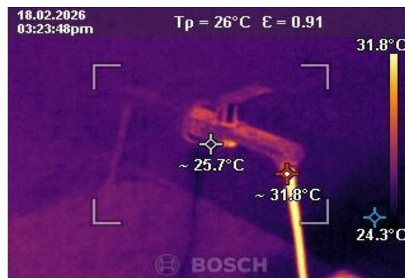
Figure 3 Shows Water Tap Leakage
