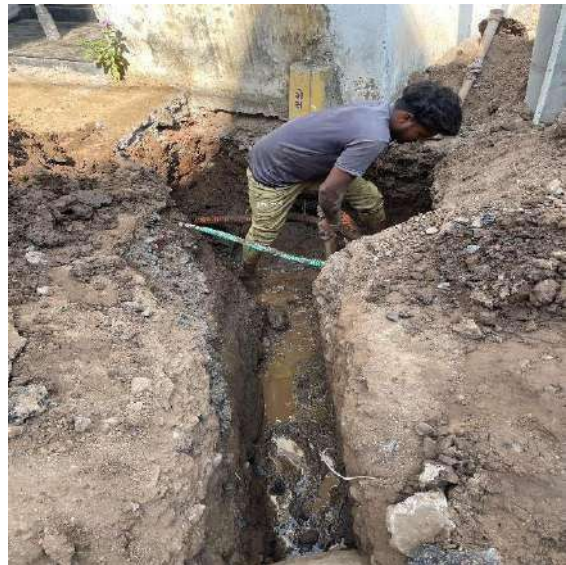
Fig 4.3 Drainage Pipe Leakage
