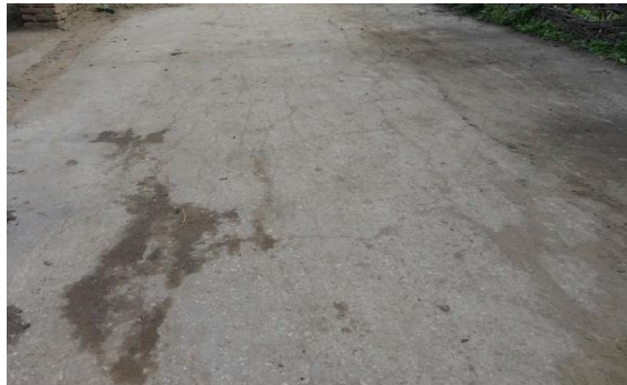
Distressed Concrete Pavement
