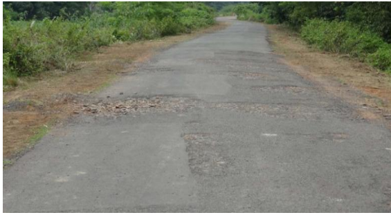
Distresses in a Bituminous Pavement
