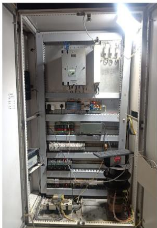
New Electric Panel
