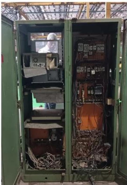
Old Electric Panel
