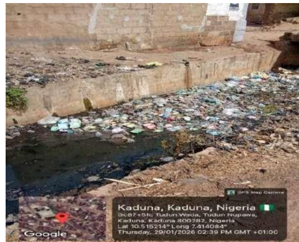
Plate 5: Waste disposal into drainage channels in Tudun/Nupawa
