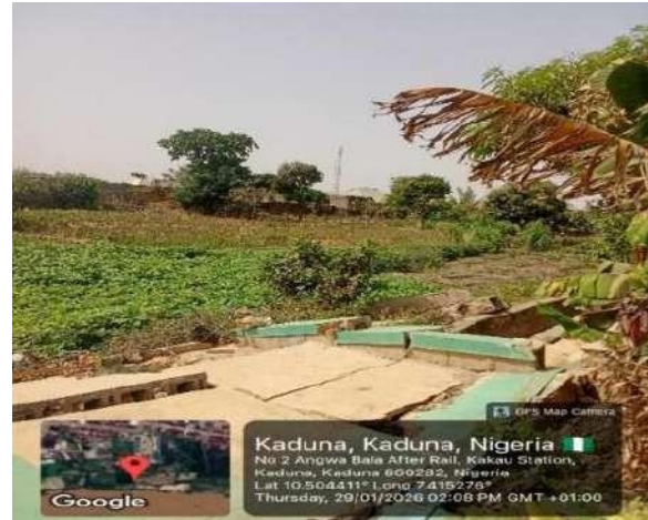
Plate 4: Dilapidated Fences in GSS, Richifa T/Wada
