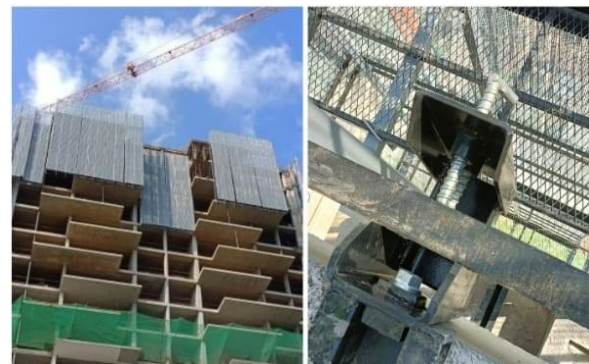
Fig..1 Images of Installed Balcony Cage system
