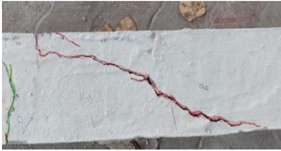
FIG 9: CRACK PATTERN OF BEAM
