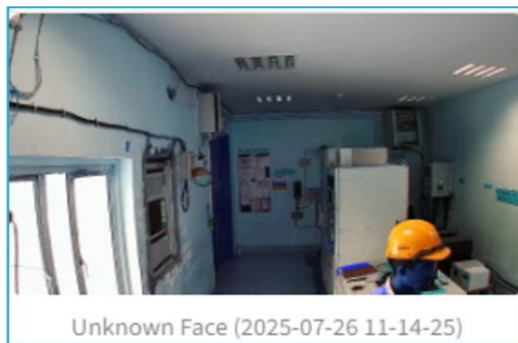
Figure – 4: Authorised Person Check
